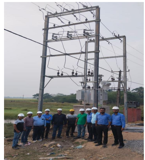
Figure 1: Voltage regulator installed in Bhadrak
