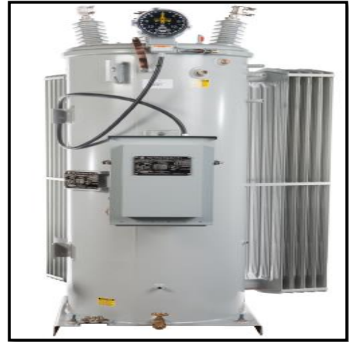
Figure 2: Pole mounted voltage regulator
